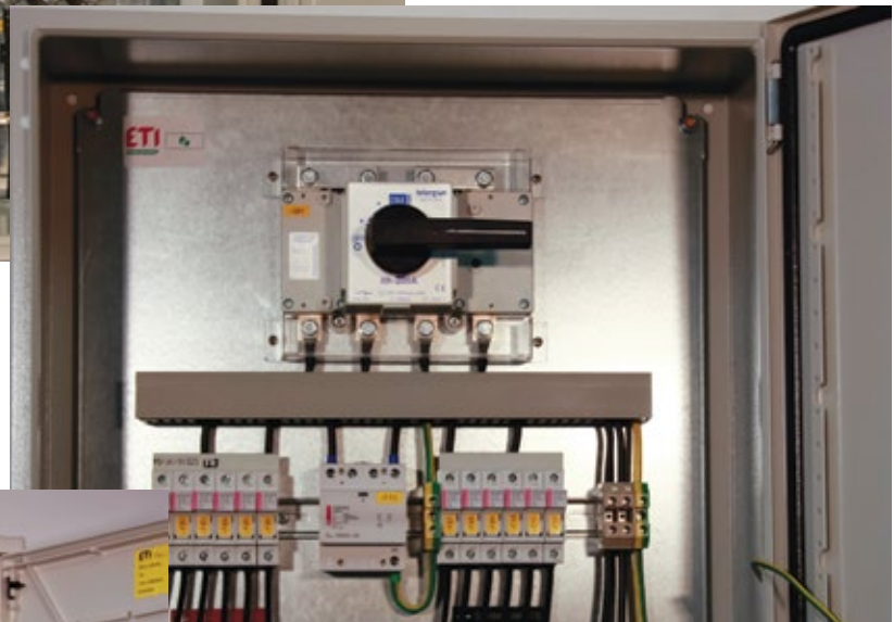
DC junction box (CH gPV fuses)
